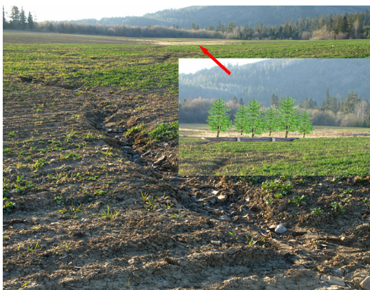
Fig. 11. The sloppy parts above the Jewish cemetery. Construction of waterholding measures on waterlogged farmland – dikes, tree planting (April 20, 2011, photo: J. Slivinský).
