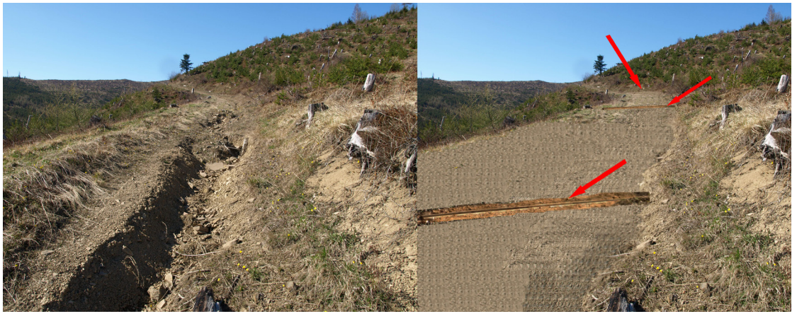
Fig. 8. Working forest road - diverters, local slope correction (left – present state; April 20, 2011, photo: J. Slivinský, right - suggestion flood measures)
