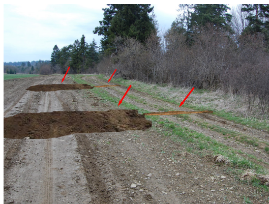
Fig. 12. Proposed measures on unused unimproved agricultural road above the Jewish cemetery – absorption ditch and hoeing of road surface (April 20, 2011, photo: M. Janiga)
